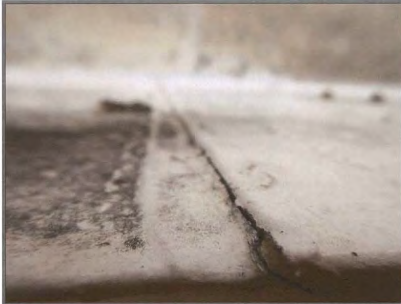
Soldered joint with a fracture near the center of the west-facing portico.
