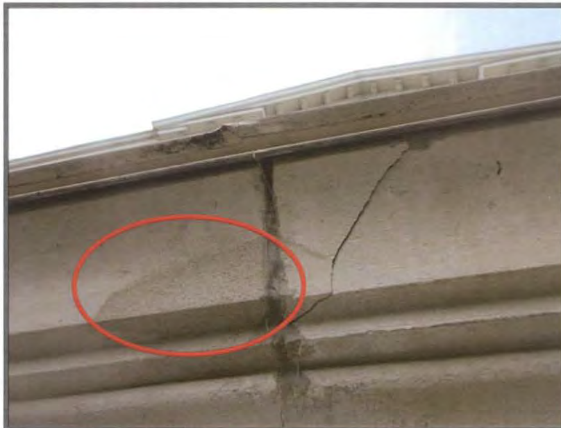
Fracture without a sealant repair on the north-facing portico. Also, note the previous composite repair (circled).
