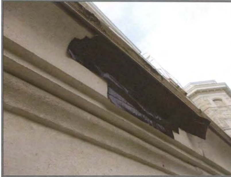
Tape applied over a fracture with a sealant repair on the north-facing portico.
