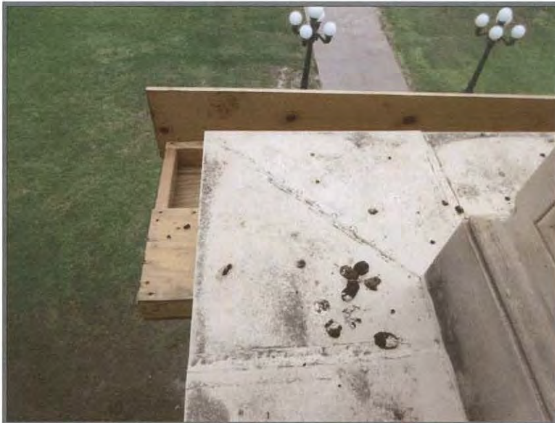
View of the top side of the soldered metal panels where the missing piece of stone cornice is located.
