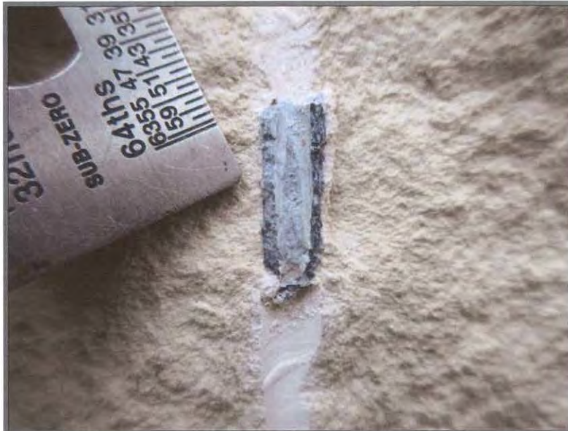
Epoxy residue at a fastener location on the piece of stone cornice.
