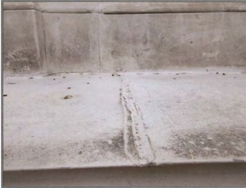
View of a soldered joint without any separations.
