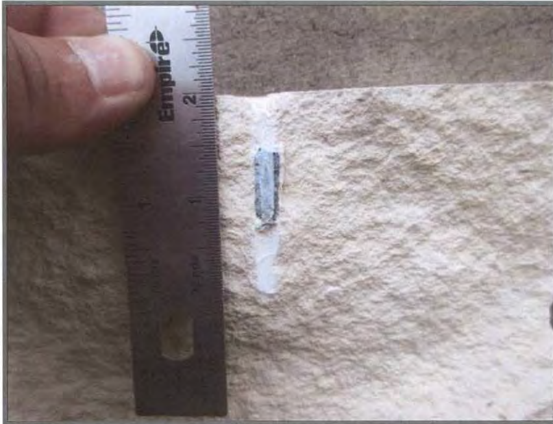
Prior fastener location on the piece of stone cornice. Note epoxy residue.
