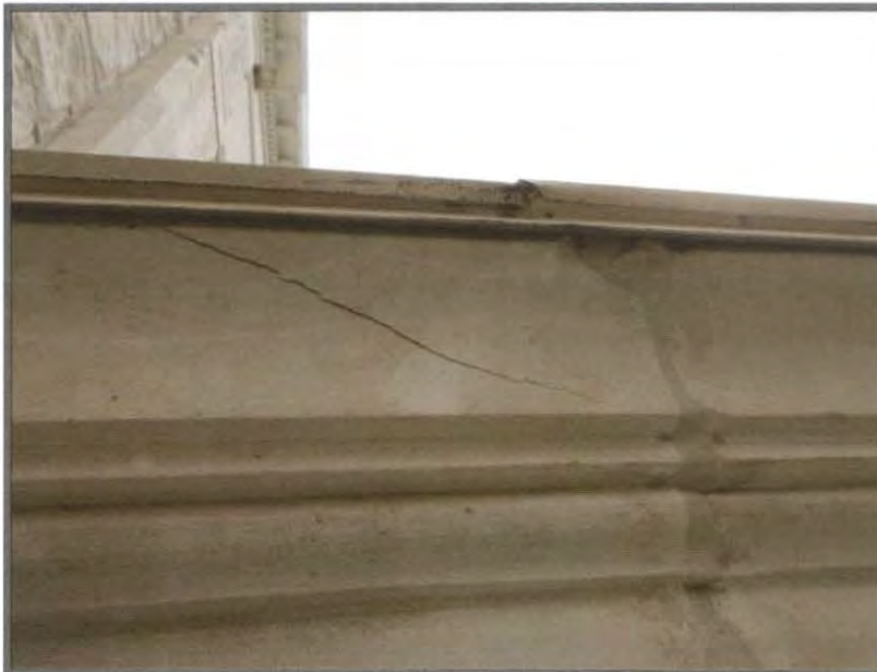
Unsealed fracture on the west-facing portico.
