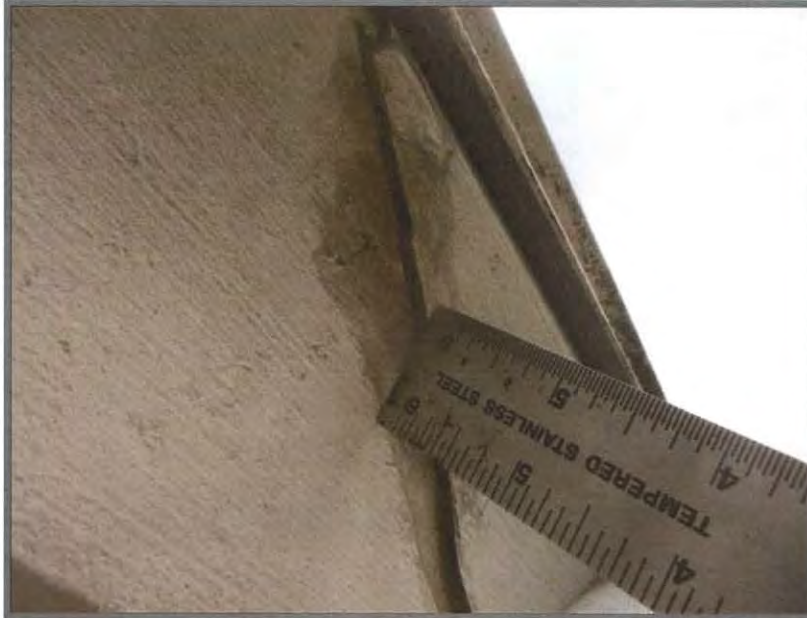
Close-up of the fracture in the previous photograph.
