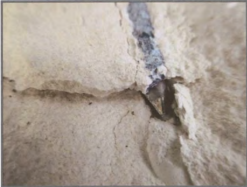
Close-up view of the fastener in the previous photograph.
