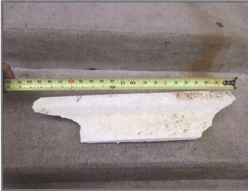
View of the exterior side of the piece of stone cornice that reportedly fell from the west-facing portico.
