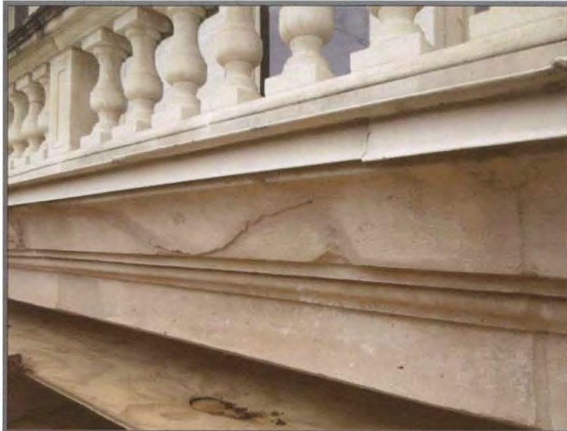
Sealed fractures on the west-facing portico.
