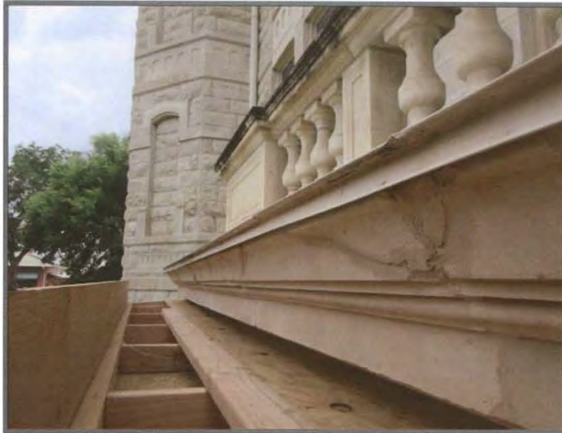
Sealed and unsealed fractures on the west-facing portico.
