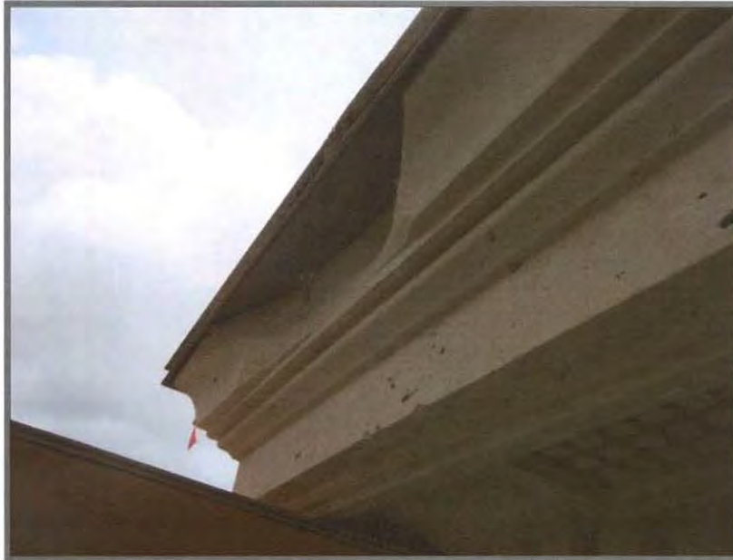
Missing piece of stone cornice on the west-facing portico. Note exposed fasteners.
