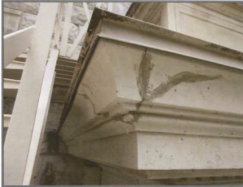
Fracture with a sealant repair on the north-facing portico.
