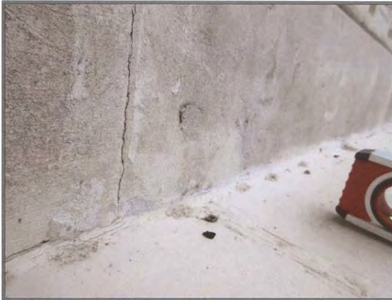
Sealant along the vertical and horizontal interface on the west-facing portico.
