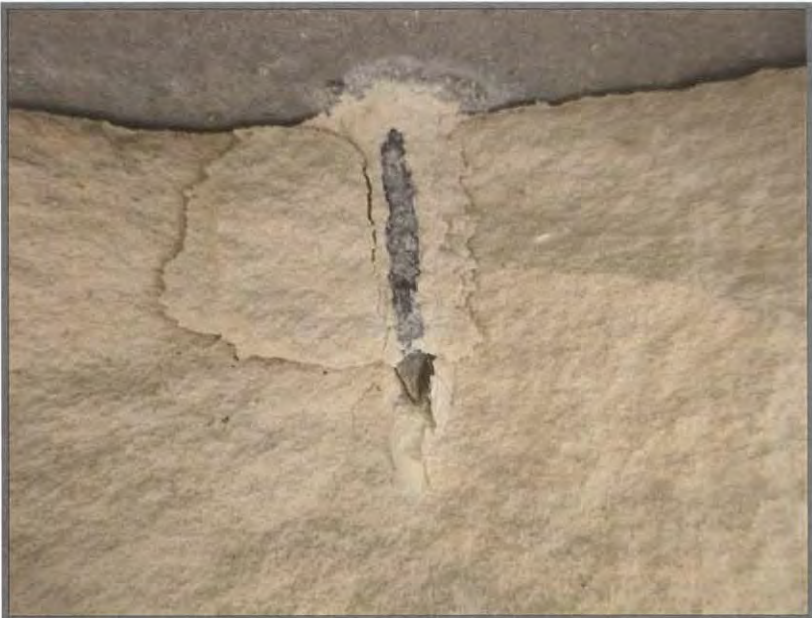
View of an exposed fastener and epoxy residue. Note absence of corrosion to the fastener.
