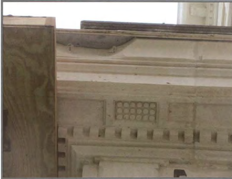
Missing portion of the stone cornice on the west-facing portico.
