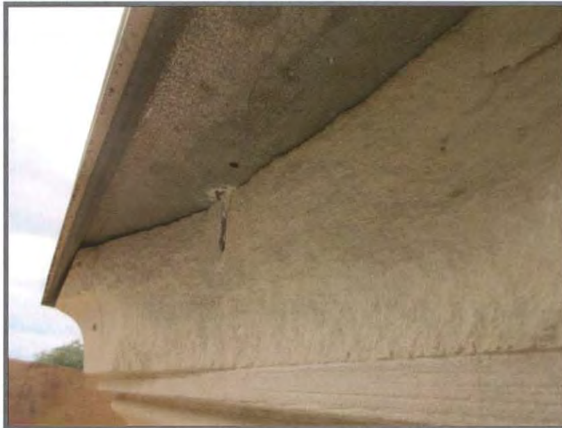
View of the fracture location. Note clean exposed stone.
